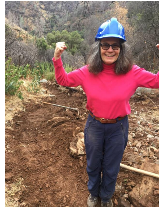
Board member Ursula Stock celebrating construction of a water diversion channel on a badly eroded road in the Hite’s Cove area.
